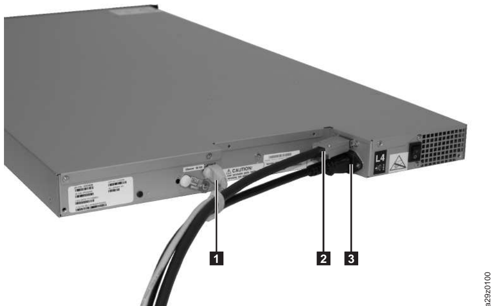
Figure 31. Interface cable connection
