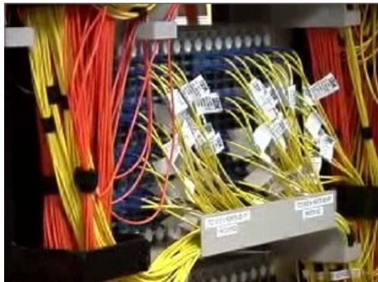
Close-up of FICON cables in a patch panel
