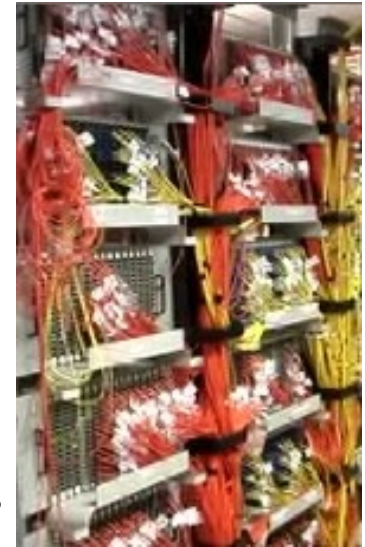
Patch panel with FICON (yellow) and ESCON (orange) cables
