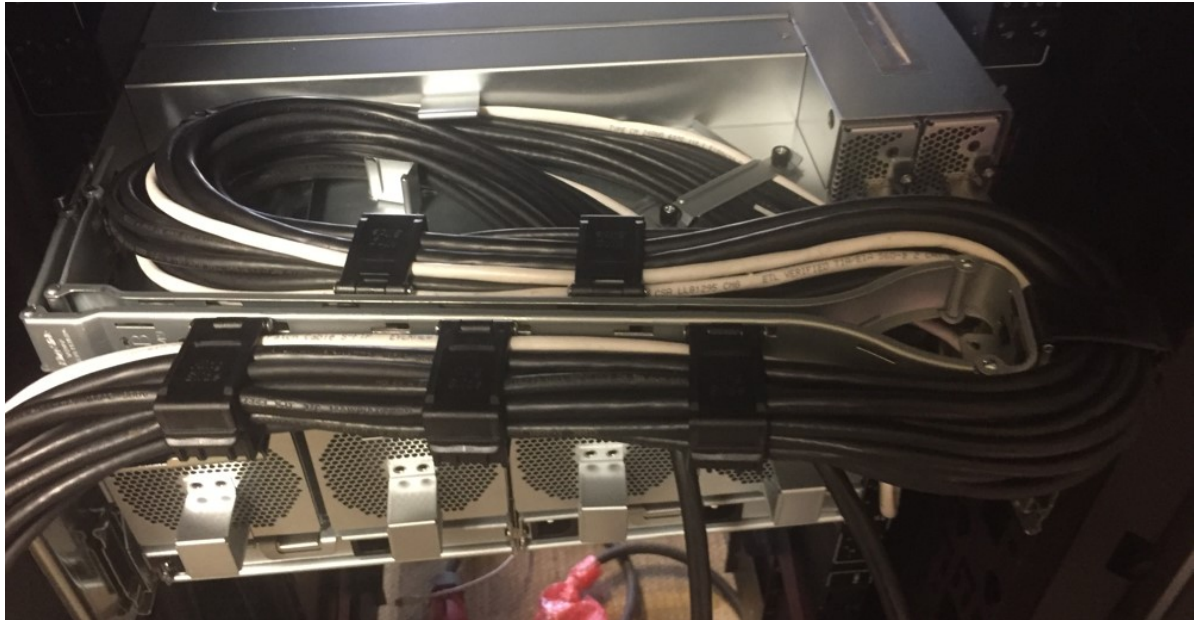
Figure 57. Cables routed through CMA baskets
